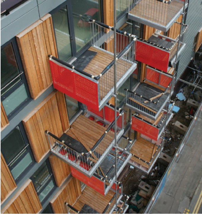
3.22 and installed Mar 2007
